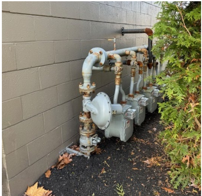
Exterior Gas Main Shutoff
