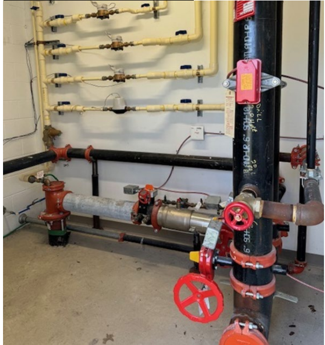
Interior Water Main Shutoff
