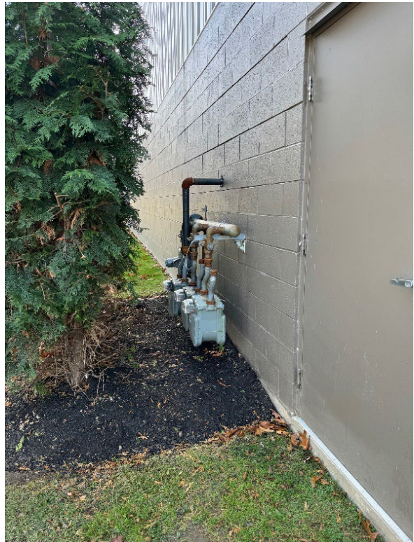
Exterior Gas Main Shutoff
